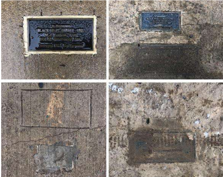
Title: Commemorative Plaques in the Greenwood District, missing or damaged.
